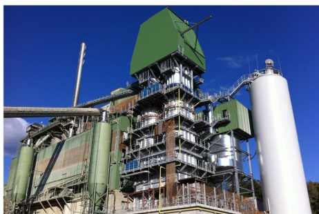
Qualical PFR Kiln in Calcis Group
